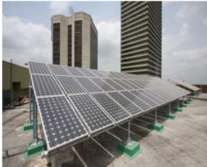
Figure 192. Solar Panel system installed on roof top can reduce carbon footprint
